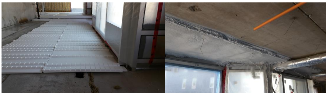
Figure 3. Thermal proofing of the cantilever balcony: polystyrene boards placed on top (left photo) and the urethane sprayed underneath (right photo)
