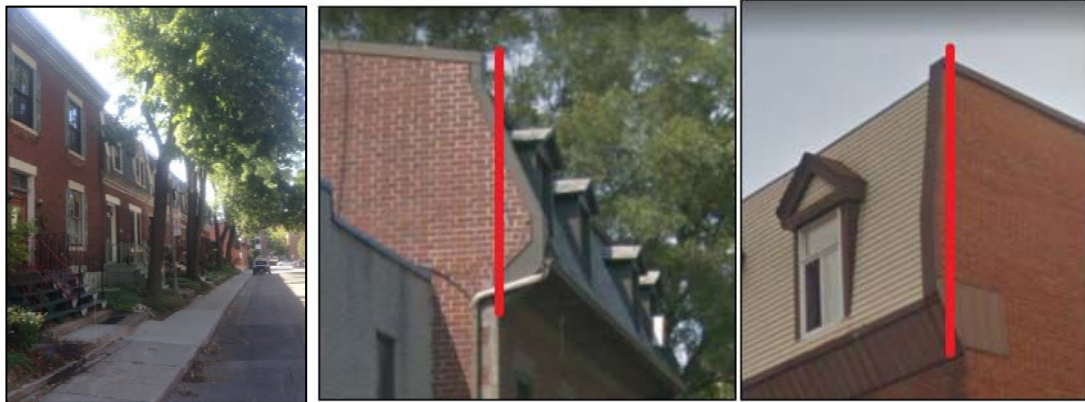
(a) (b) (c) Figure 2: Typical URM-B1 houses: (a) in Westmount, (b) with real mansard roof, (c) with false mansard roof.
