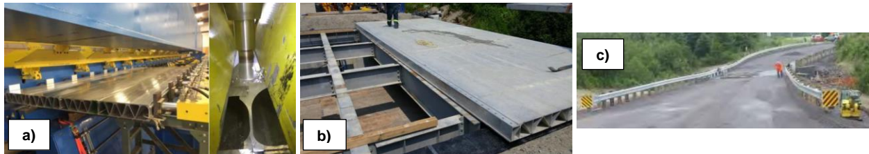
Figure 1: Aluminium bridge deck a) Extrusions joined by FSW b) Installation c) Final product (Beaulieu and Internoscia 2015)
