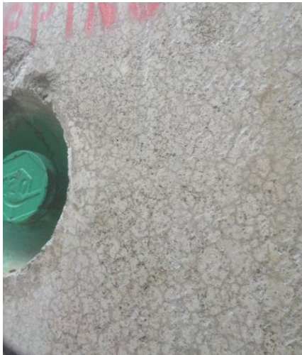
Figure 1: Box culvert surface for Kaskawan Creek, 2015, 96-hour cure by wet burlap and sprinkler
