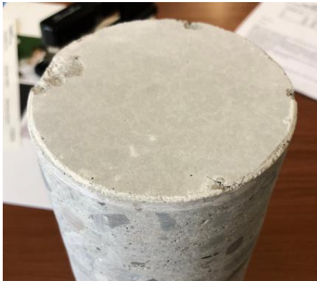
Figure 3: Core sample taken from the box unit from Meatbird Creek Culvert in dry state
