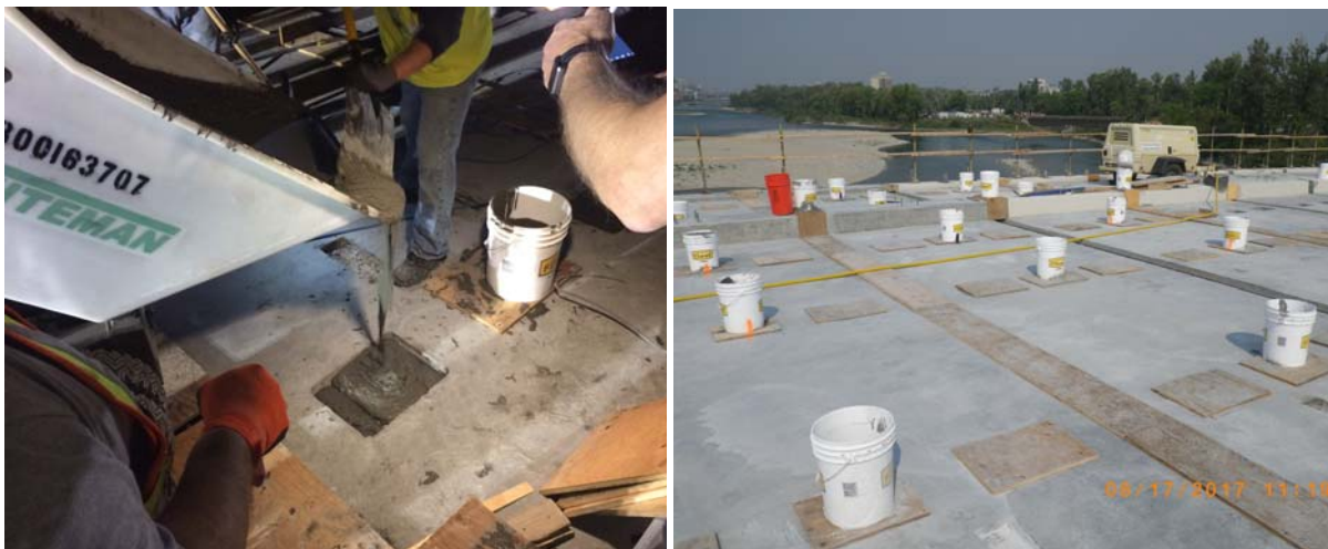
Figure 10: A) UHPC placement in a shear pocket and B) Top formwork and head buckets after placement
