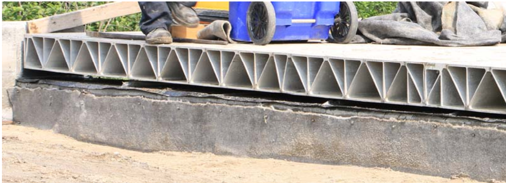
Figure Error! No text of specified style in document.-1 : AlumaBridge aluminium deck used for the construction of a short span bridge at St-Ambroise, QC, Canada; July 2015 (From the photo archive of the Aluminium Research Centre – REGAL).
