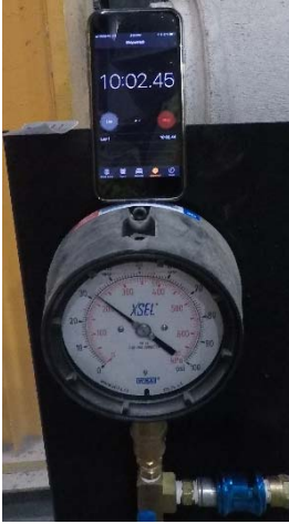
Figure 7 Pressure Gauge and Time Measurement
