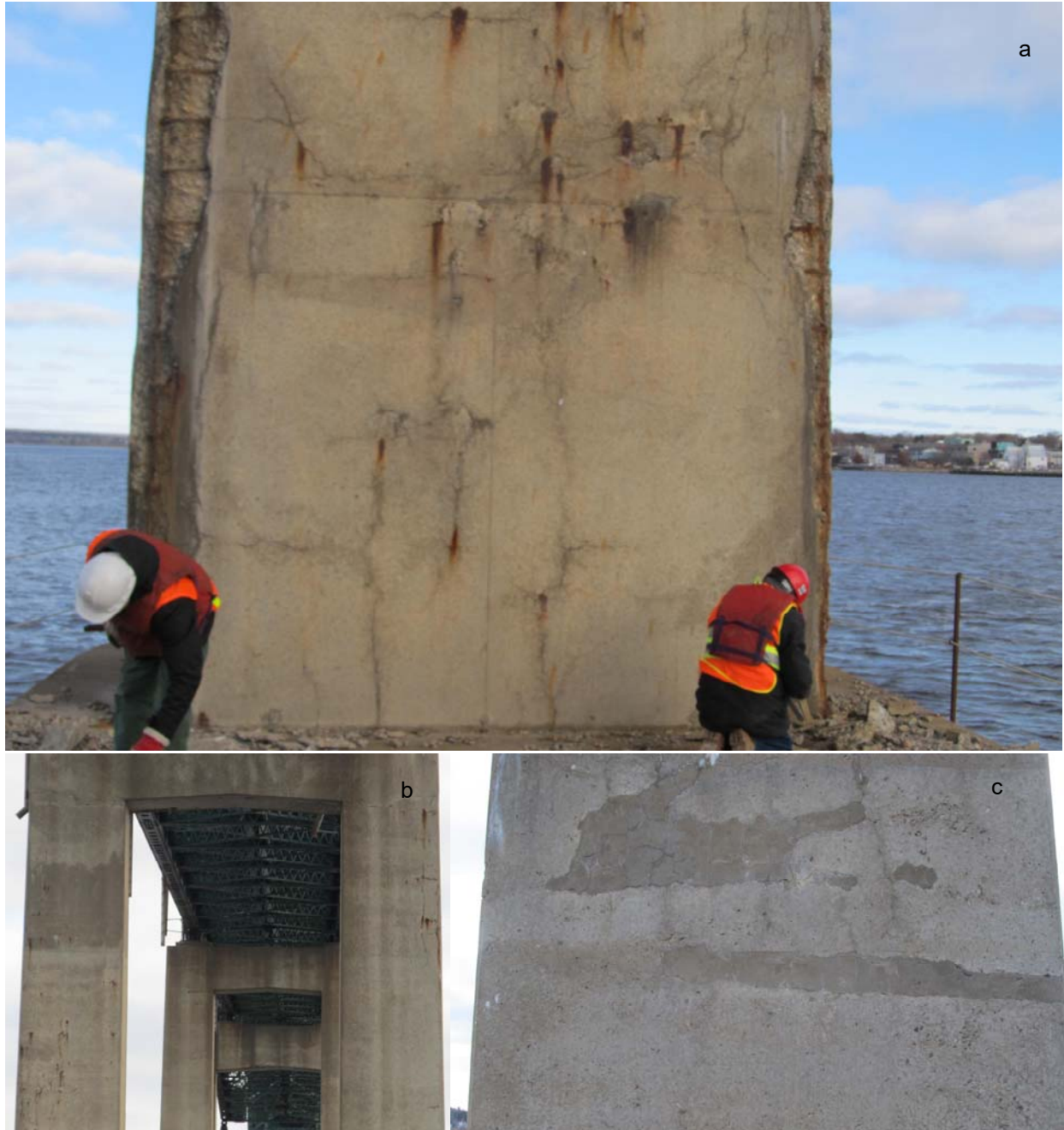
Figure 3: Examples of Deterioration Observed. a) Corrosion and Corrosion-Induced Loss of Section, Pier 11; b) Cracking with Visible Corrosion Product Seepage, Pier 13; c) Improperly Repaired Honeycombing, Pier 11
