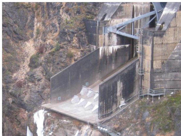
Figure 3 View of REs Installed on SW2 Chute
