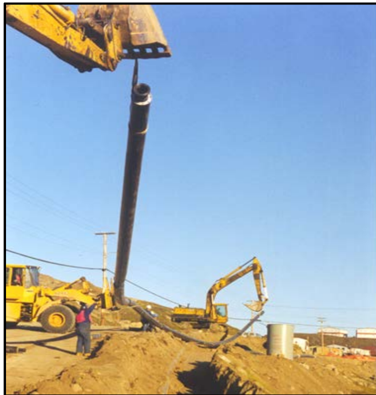
Figure 7: Iqaluit's water and sewer system pioneered the use of insulated HDPE pipe
