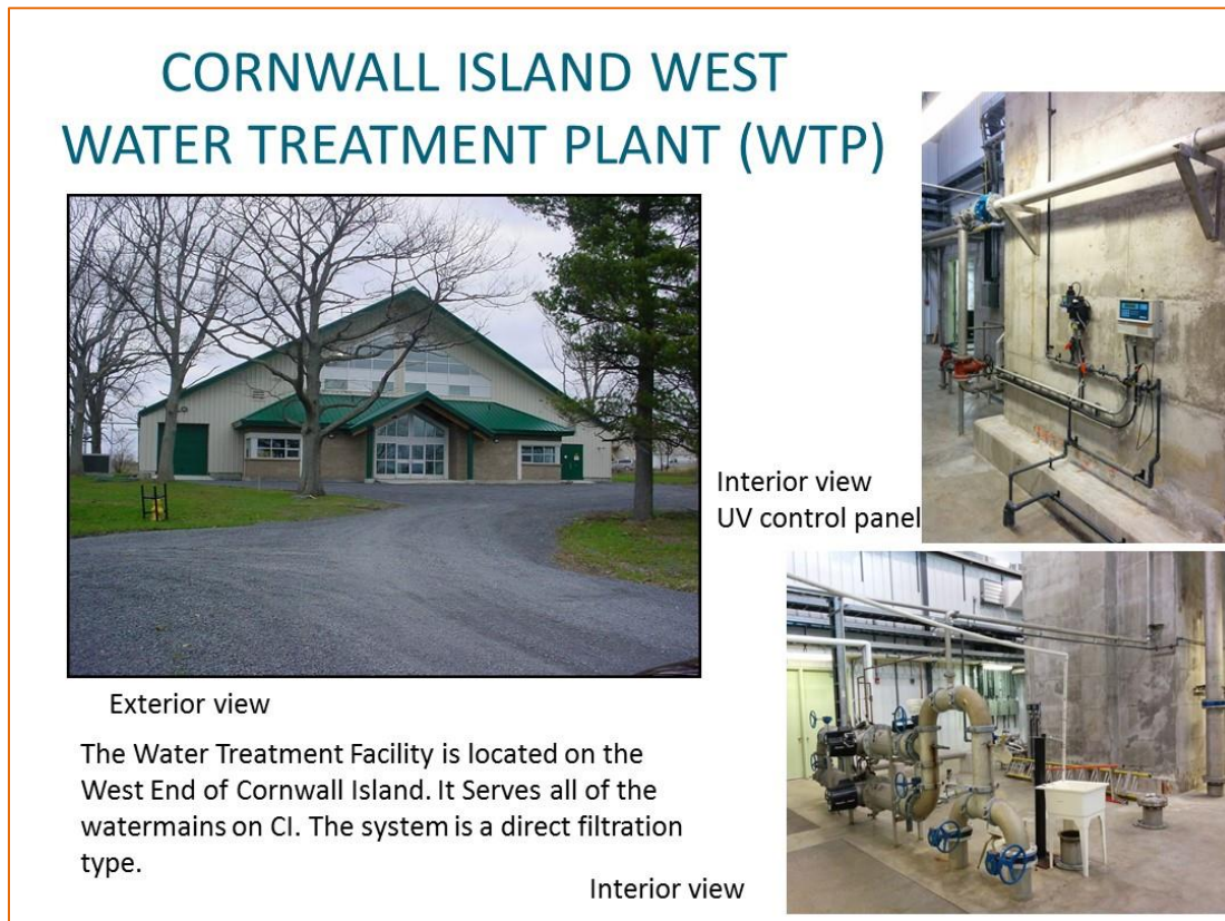
Figure 2: Akwesasne Cornwall Island Water Treatment Plant (Source: Mohawk Council of Akwesasne)
