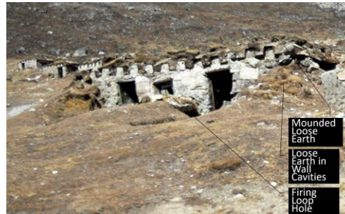
Figure 1: Rear view of a typical concrete firing bunker at a remote location ("Indian Army for Better Frontline Infrastructure," 2014)
