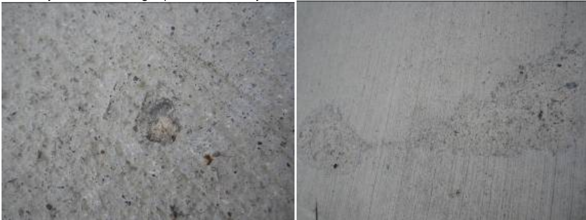
Figure 10: Minor pop-out (left) and scaling (right) occurrence in mixes
