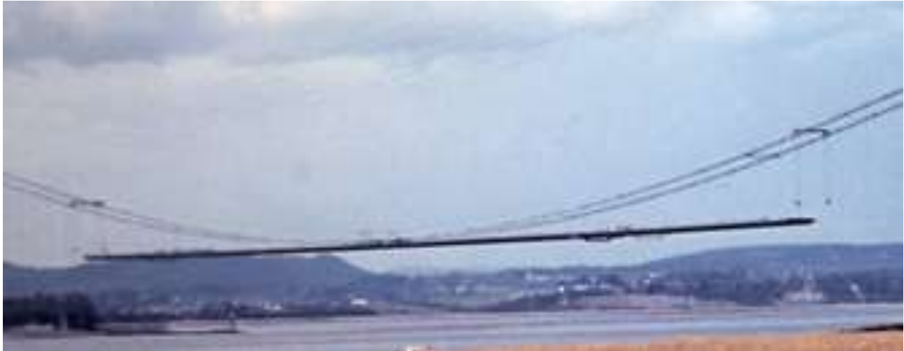
Figure 3: Assembly of the deck segments of the first Severn Bridge, UK (Spicer, 2011).
