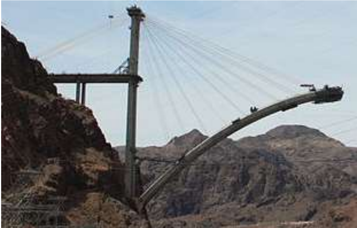
Figure 2: The construction of the Hoover Dam Bypass Bridge using the unidirectional cantilever construction method (Wikimedia, 2010).
