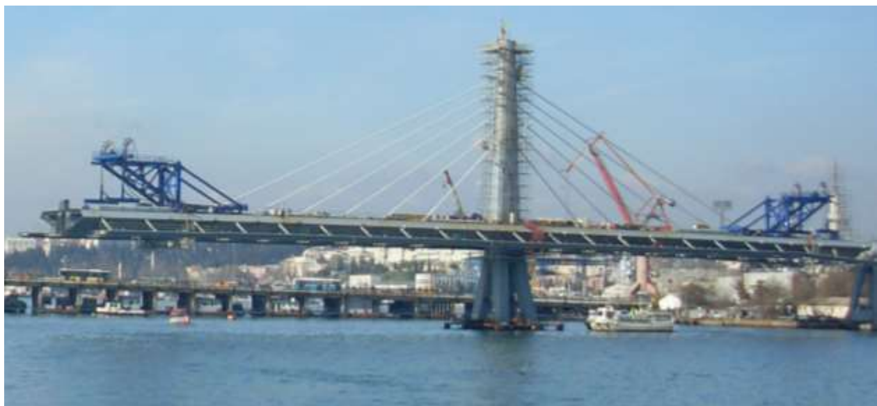
Figure 1: Construction of the İstanbul - Golden Horn Metro Bridge using the balanced cantilever method (WikiPicture, 2013).
