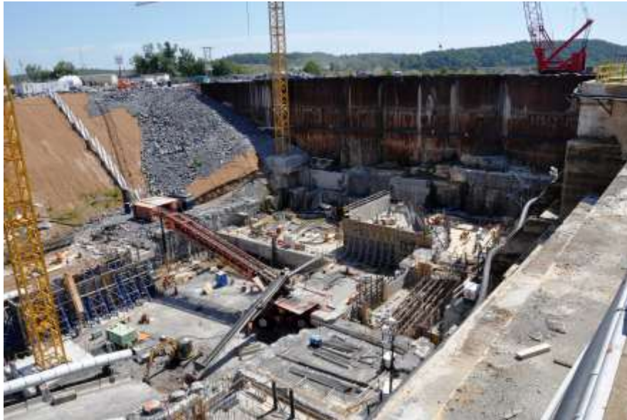
Figure 1: A cellular sheet pile cofferdam used to construct a lock in-the-dry in Nashville, Kentucky, USA (Tucker, 2012).
