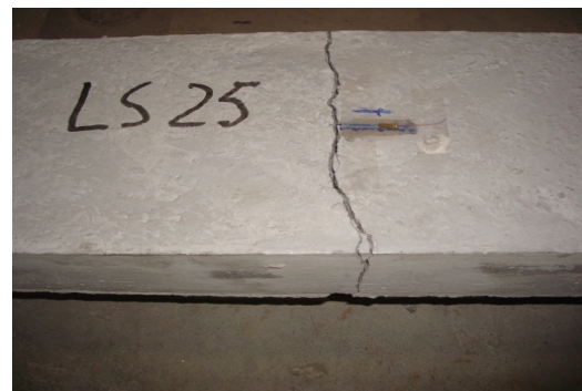
Single crack in LS-SCC
