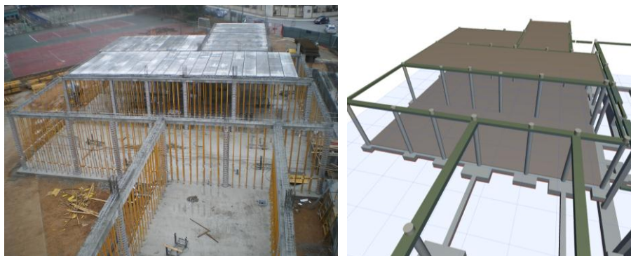
Figure 7 & 8: Progress of the works for as-built: structure of the building (left) and render image (right)
