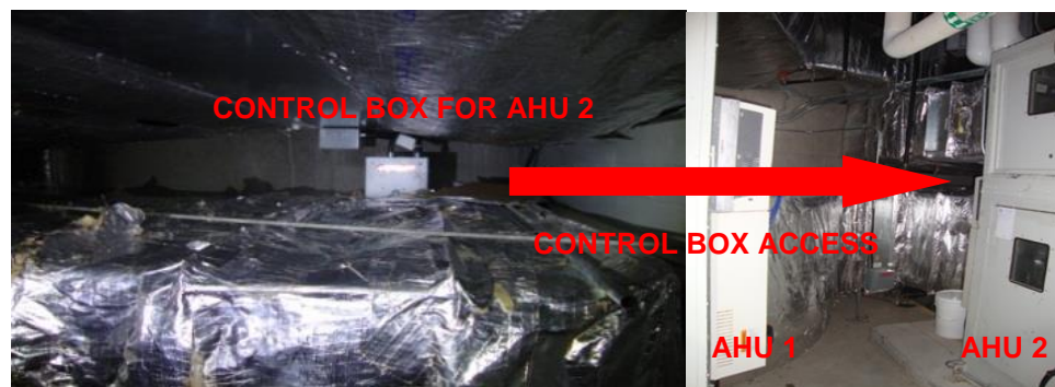
Figure 5: Restricted Access to the Control Box of the Air Handler Unit (AHU).
